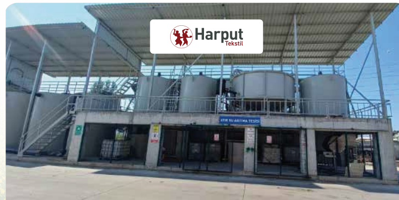
Gökçeköy Weaving Facility /wastewater treatment plant
